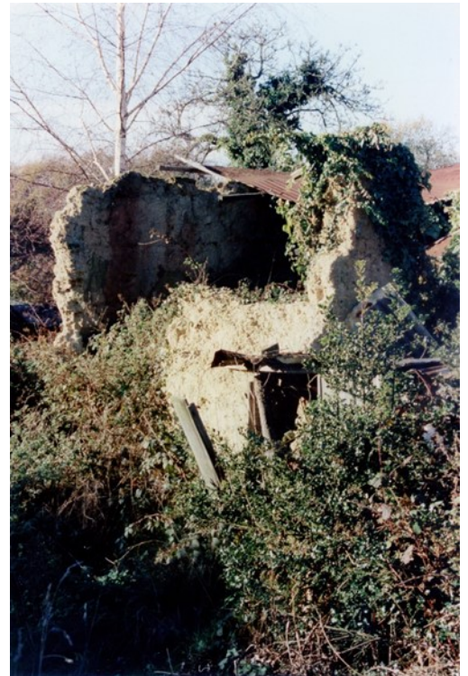
The remains of a cob wall at Cripplestyle, once a shop run by Keturah Butler Remains like these used to be dotted around the parish!
